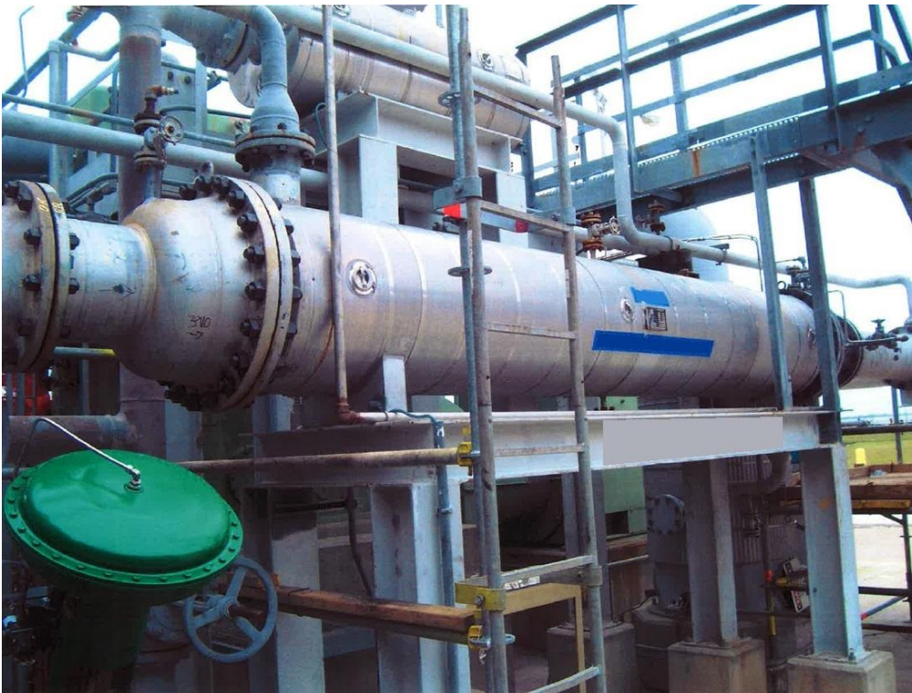
Figure 1: Photograph of heat exchanger to be replaced
